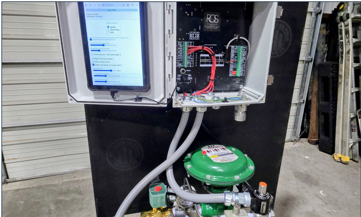
THE TRIM UP CLOSE — ASCO ESD, PARKER PILOT & MAIN SOLENOIDS, FLOPRO D2T, REGULATORS & GAUGES · TOUCHSCREEN IN OIL HEATER TREATER MODE
